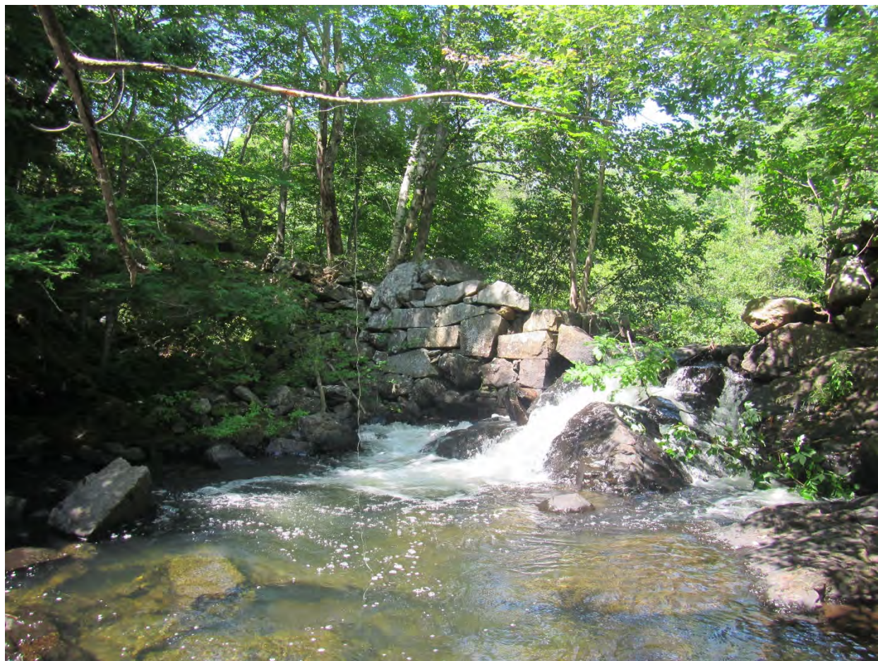
Figure 49. The Powder Mill Dam ruins. Granite blocks dislodged from the dam are visible in the channel in the foreground.
