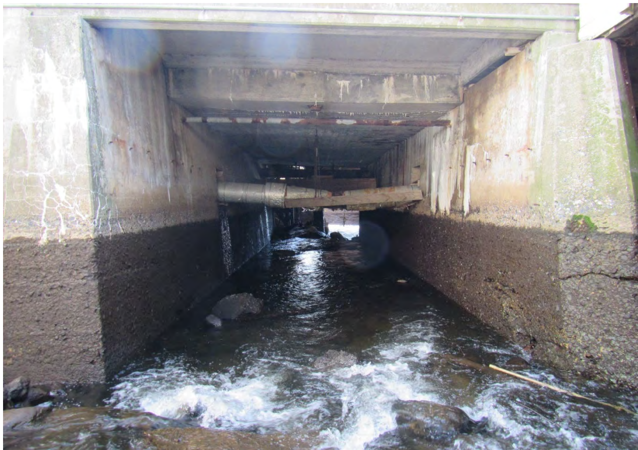
Figure 27. View downstream through north span of Main Street bridge in drawn down condition, May 8, 2018. Stain lines indicate normal pool elevation.
