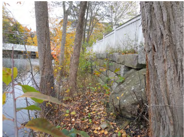
22) 51 Mechanic Street and parking lot – gravity retaining wall along shore is rotated with some misaligned elements
