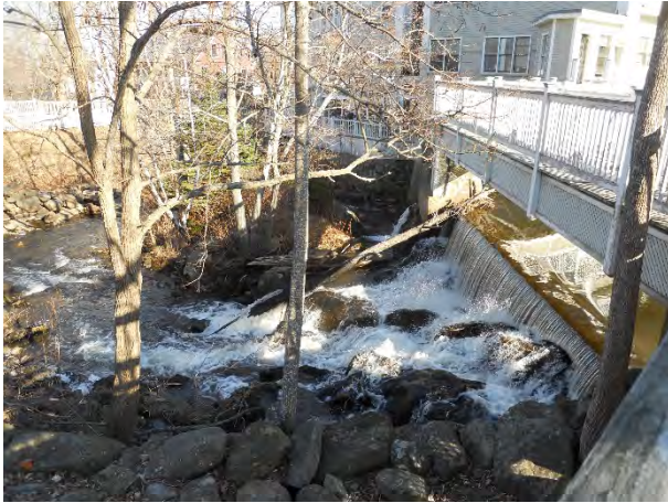
13) Knowlton Street Dam (north spillway), 51 Mechanic Street and pedestrian bridge to 2 Knowlton Street
