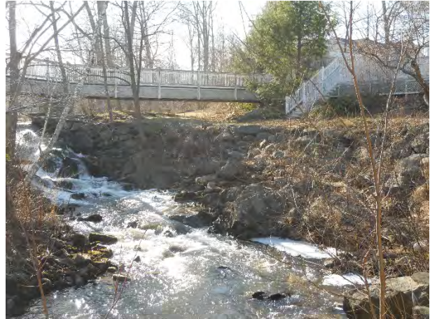
14) Knowlton Street Dam (north spillway), pedestrian bridge to 2 Knowlton Street, shoreline downstream river left (possible fish passage zone)
