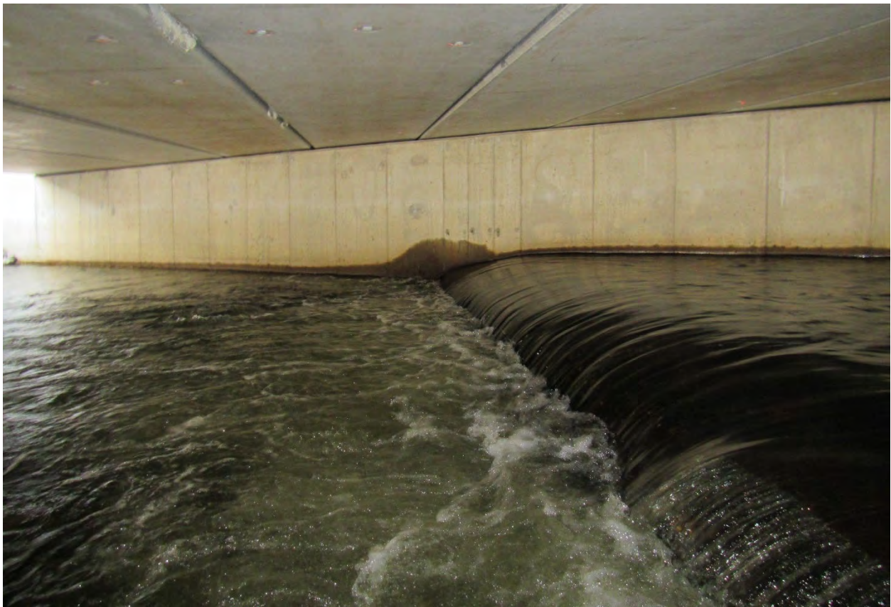
Figure 32. View across channel beneath Washington Street bridge, May 8, 2018. Concrete sewer line encasement creates hydraulic drop of approximately 9 inches.
