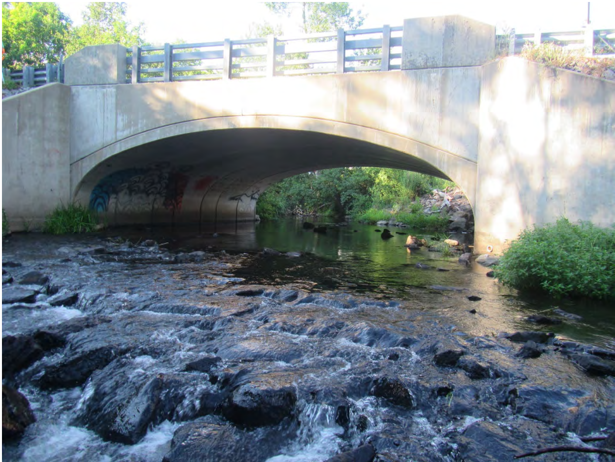
Figure 45. Looking upstream at the Washington Street crossing, A constructed grade control riffle is visible in the foreground.
