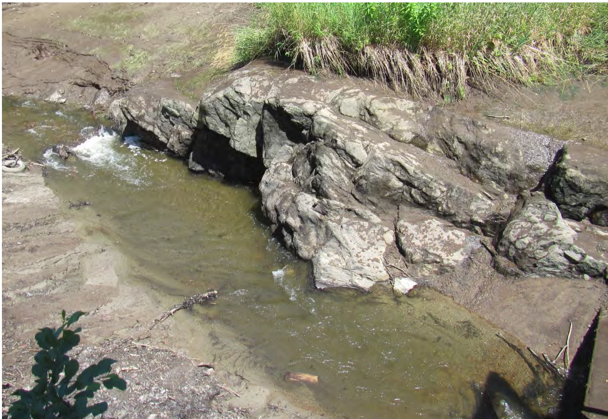
Figure 94. Photo of the channel immediately upstream of Knox Mill Dam in a drawn-down condition. The shadow of the open gate structure is visible in the bottom right corner.
