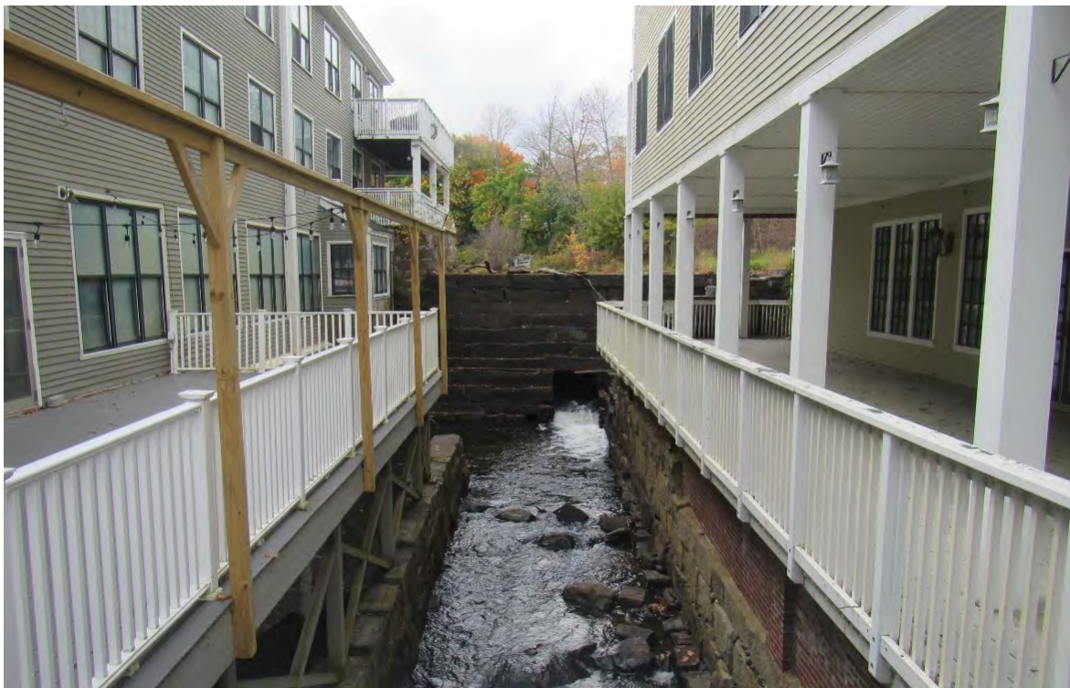
Figure 36. Downstream view of Knox Mill Dam. Previously mill buildings extended completely across the river.
