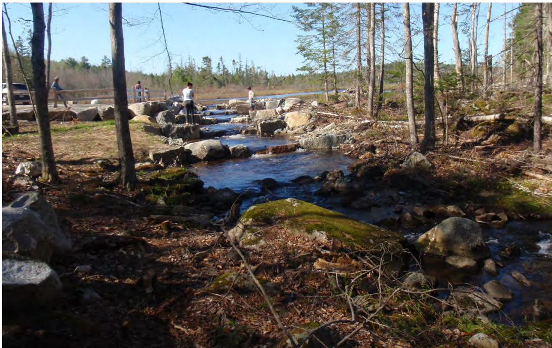
Figure 91. Examples of constructed nature-like fish passage (photo credits: Matt Bernier).
