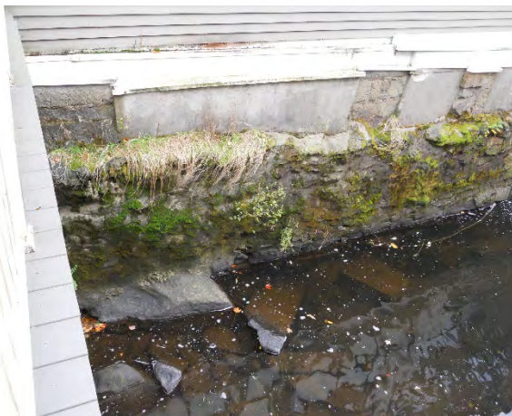
29) 32 Mechanic Street – Minor repairs are needed; dam removal may change but not significantly worsen existing conditions
