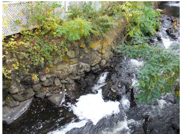
16) 51 Mechanic Street foundation – Repairs are needed; dam removal would change but not significantly worsen existing conditions
