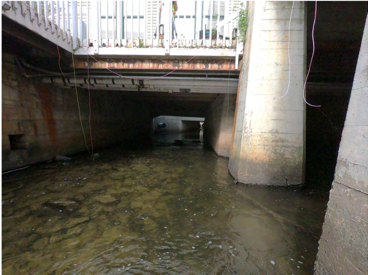
Figure 33. Looking downstream from below The Jack restaurant. The channel is walled on both sides, with numerous building footings present in the channel. The coarse bed substrate is visible in the center of the channel.
