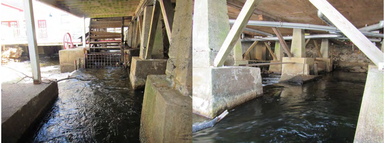
Figure 31. Looking downstream beneath the Brewster building, May 8, 2018. Relict water wheels and weirs between pier footings visible in images.
