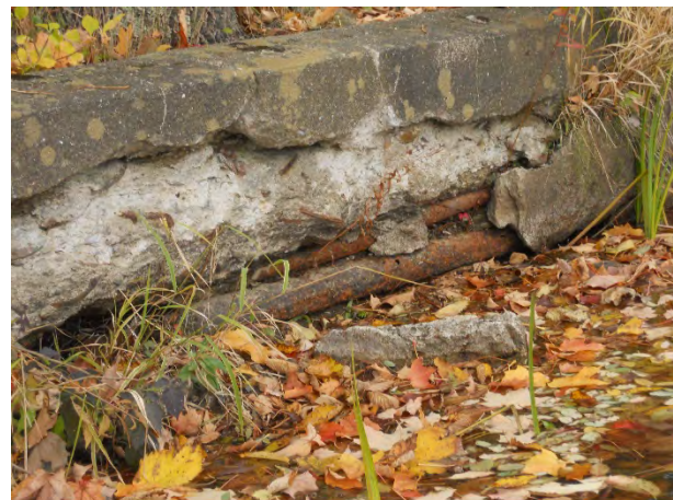
18) Knowlton Street Dam – North retaining wall (degraded)
