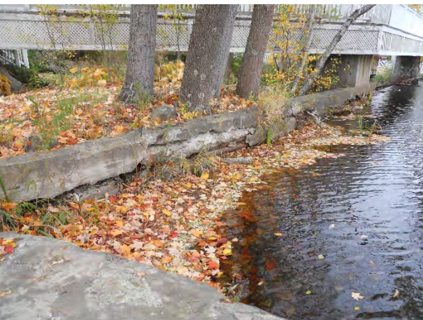
17) Knowlton Street Dam – North retaining wall (degraded)
