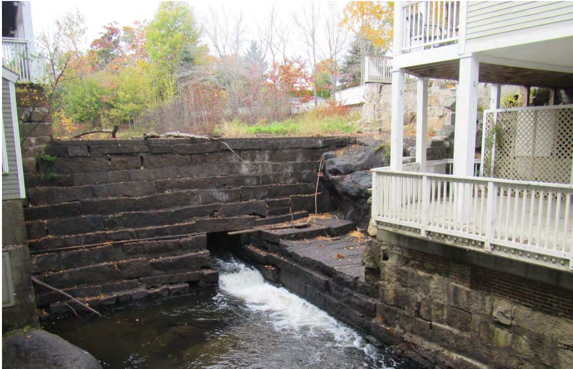
Figure 35. Downstream view of Knox Mill Dam. Previously mill buildings extended completely across the river.
