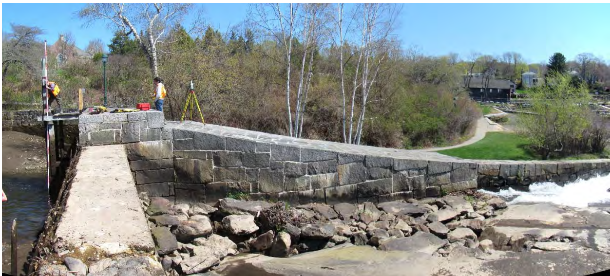
Figure 11. View of north end of spillway, the stone outflow culvert, and ledge outcrop, May 8, 2018. The seawall and Harbor Park are at the right of the image.
