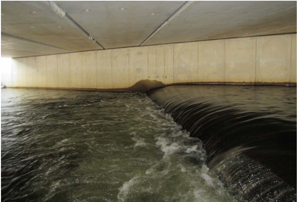
Figure 29. View across channel beneath Washington Street bridge, May 8, 2018. Concrete sewer line encasement creates hydraulic drop of approximately 9 inches.
